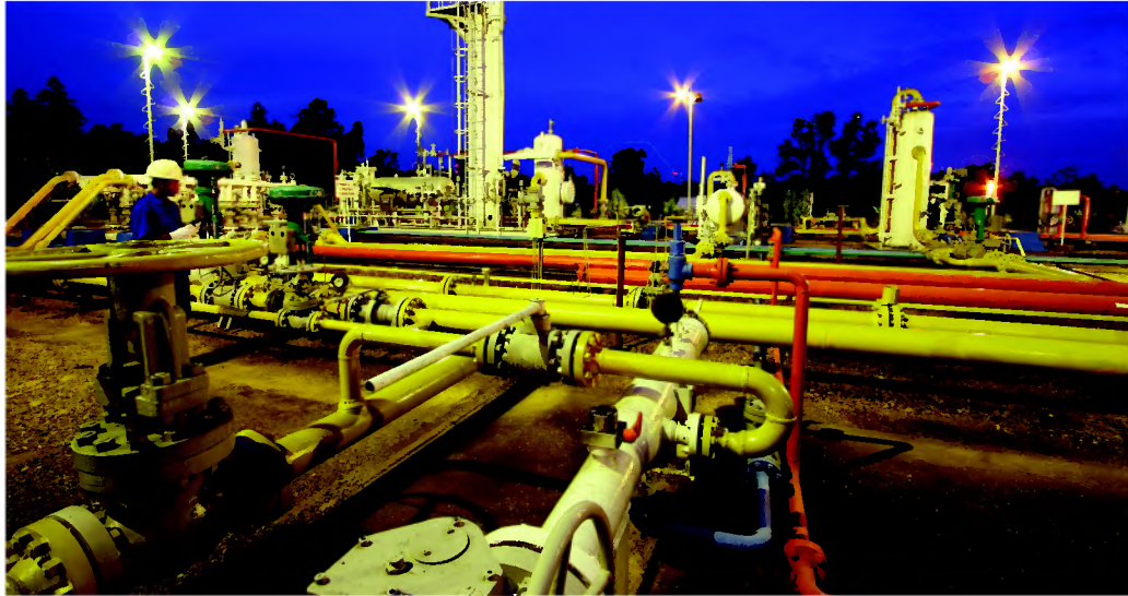
Gas Gathering Station - Medco E&P
