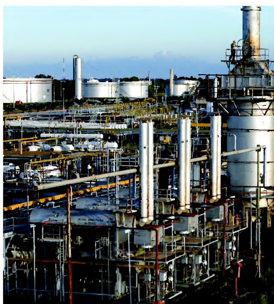
Gas Plant - VICO
