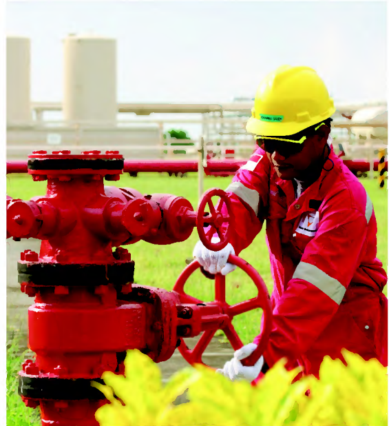
Wellhead - Kangean Energy
